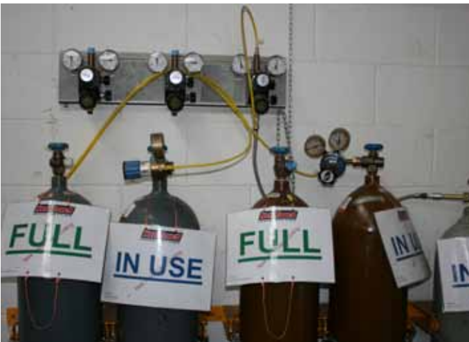
Designated locations and status labelling reduce time checking gas bottle condition.
